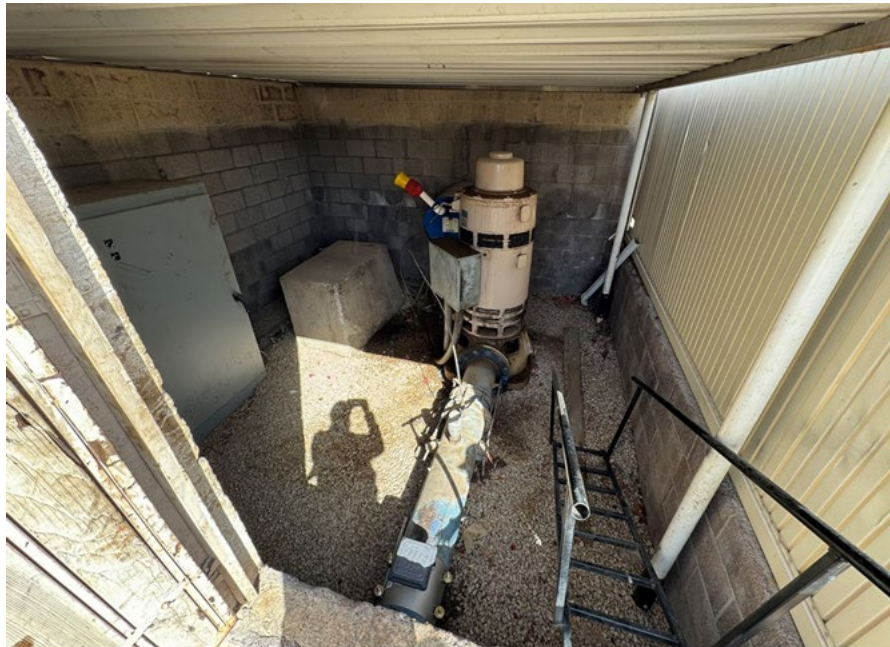
The well providing water for the Vistas Course has reached the end of its useful service life and will need to be replaced soon.
